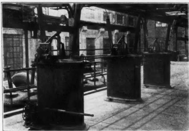
FIG. 10—60,000-VOLT TRANSFORMERS AND CIRCUIT-BREAKERS
